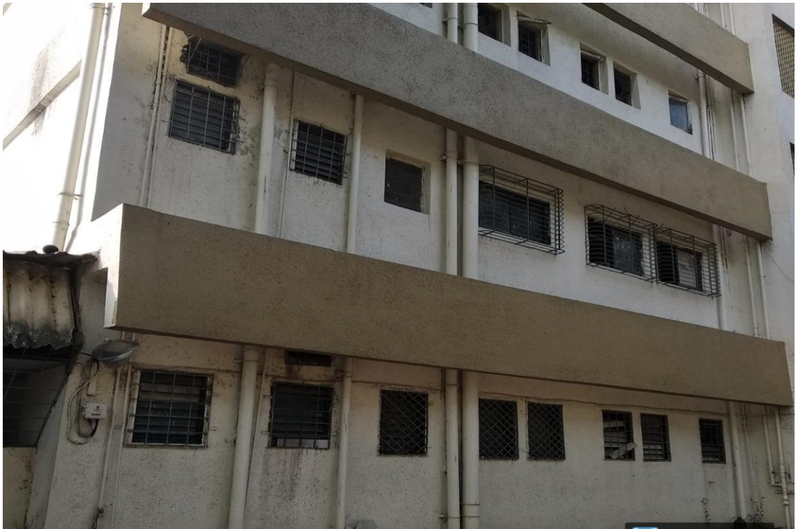
Drainage Pipe Lines
